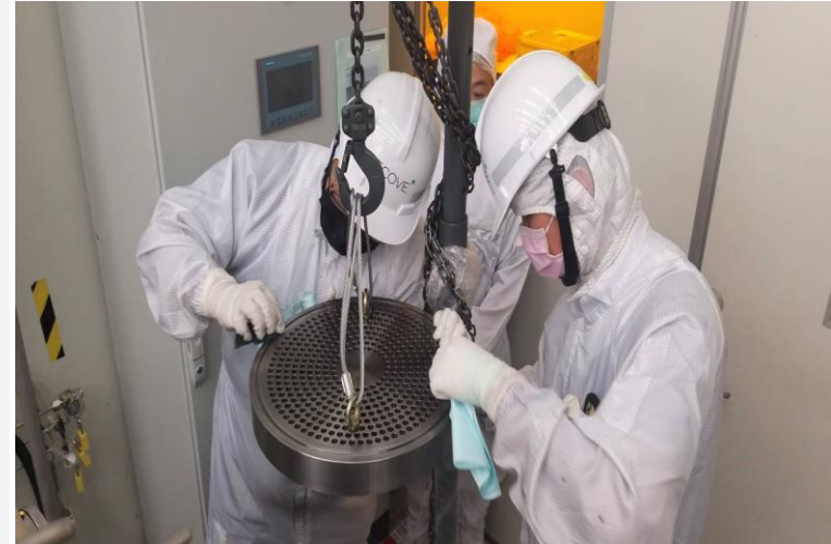
Maintenance and servicing of cleanroom process equipment
